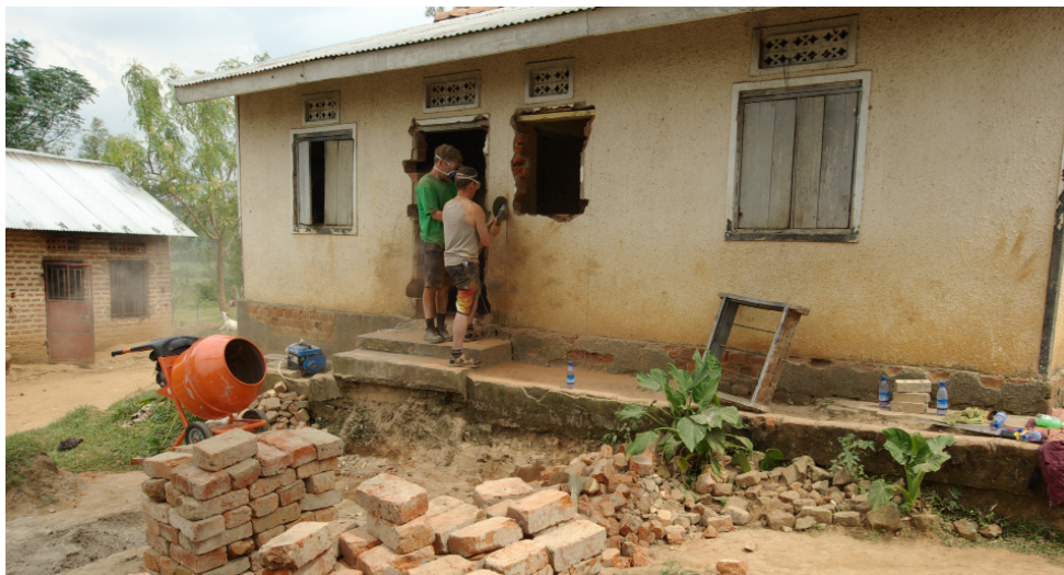
Work in progress on the back of Kukubarra House, the oldest house in the village
