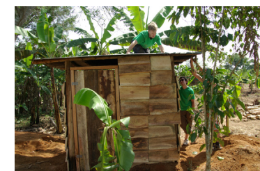
The hut over the pit latrine nears completion. It took the team a morning to complete
