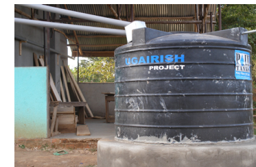
Water harvesting tank on one of the Farm School buildings
