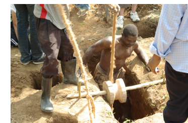
Joseph the latrine digger, emerging from the new pit dug for the elderly lady in the bush
